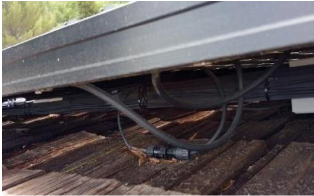
Connectors/ cables directly placed on roof or ground surface
