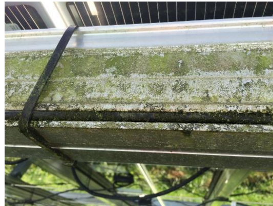
Cable permanently exposed to water
